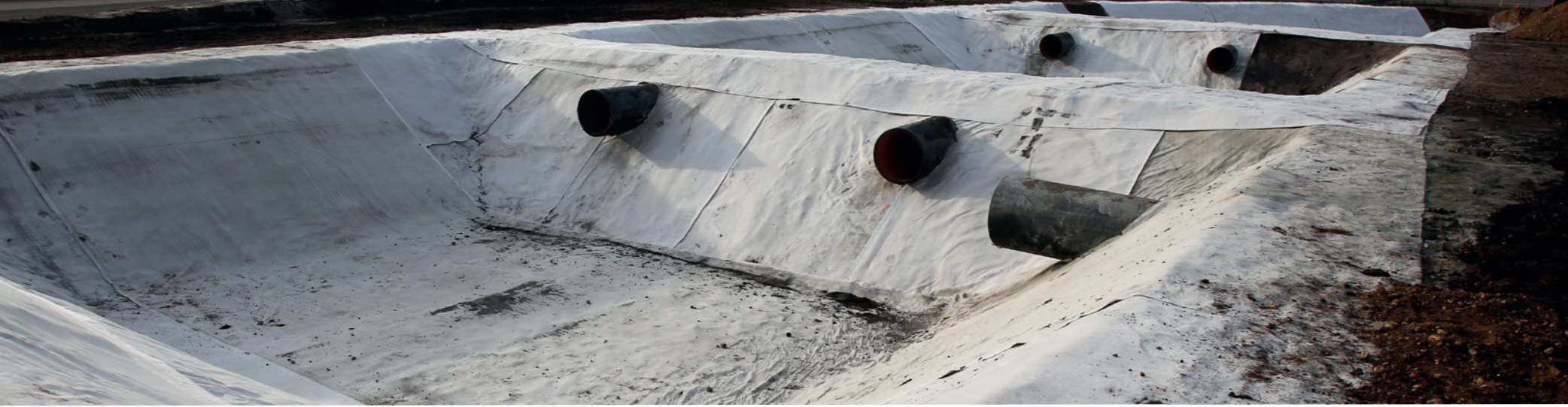
POND AND RESERVOIR LINING
